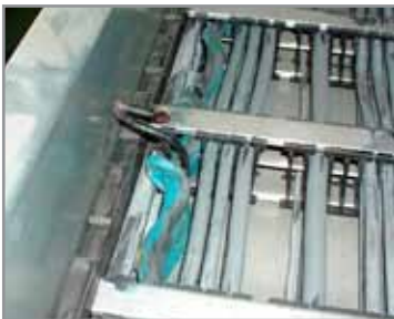
Cable failure showing entangled cables and ruptured jacket.
