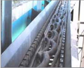
An example of corkscrewing where cables twist themselves.
